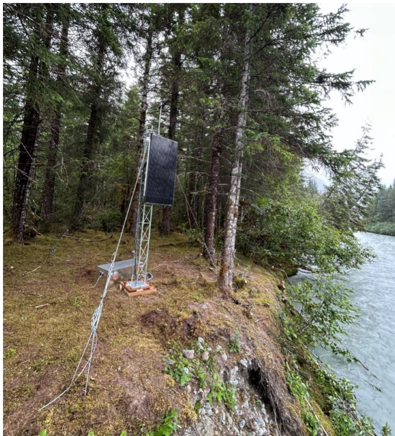
Fig. G: New river monitoring gauge installed in Herbert River at project site
